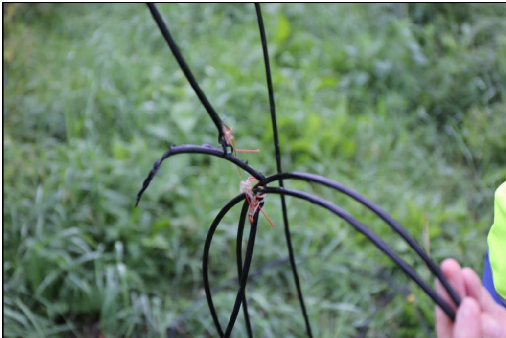
Photo No. 2: The wire ends as found following the accident.
