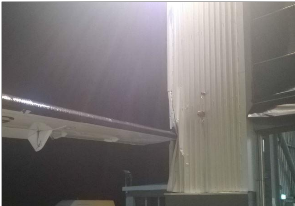
Photo No. 1: Left wing-tip impact with hangar cladding
