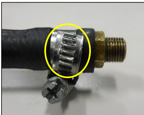
Photo No. 5: Hose clamp/clip in its tightened state, with large portion of threaded band protruding at screw head.
