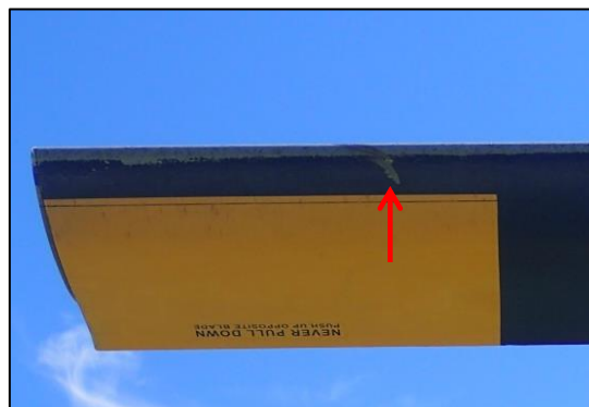
Photo No. 4: Damage on lower surface of outer section of the leading edge
